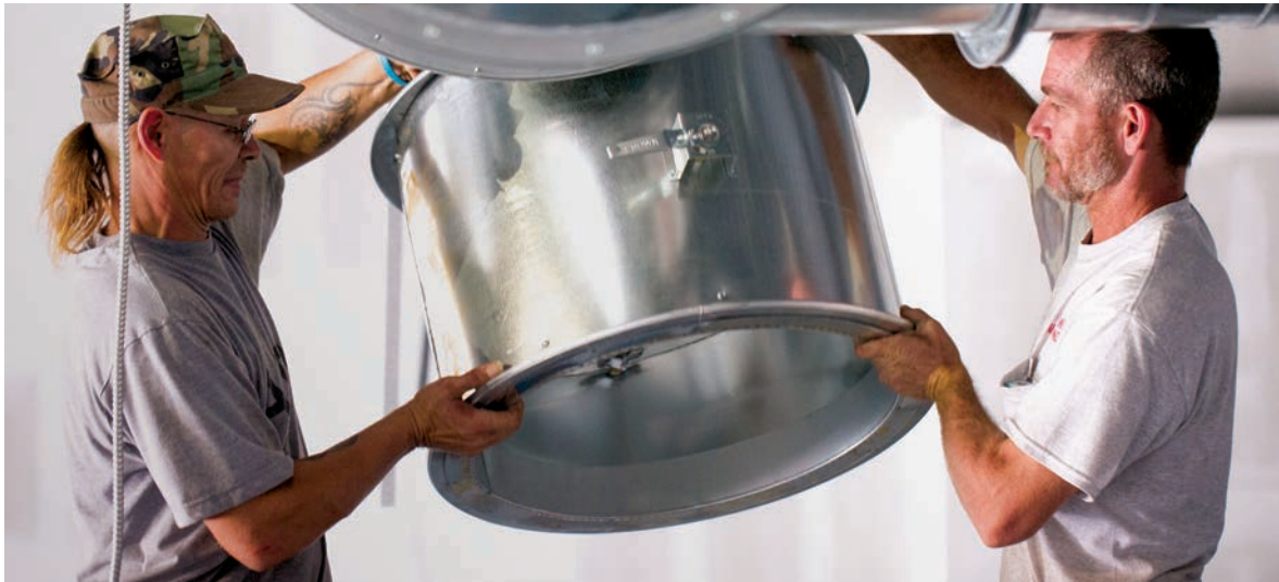
Brothers Mat (left) and Andy Grimes hoist ductwork to complete a commercial air conditioning installation.
