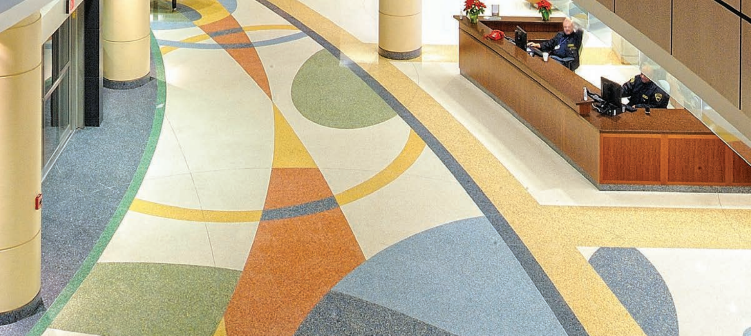
The UF Health Shands Cancer Hospital, Gainesville, Fla., features a 7,396-square-foot epoxy terrazzo floor by Artistic Surfaces that is beautiful, easy to maintain and durable.
